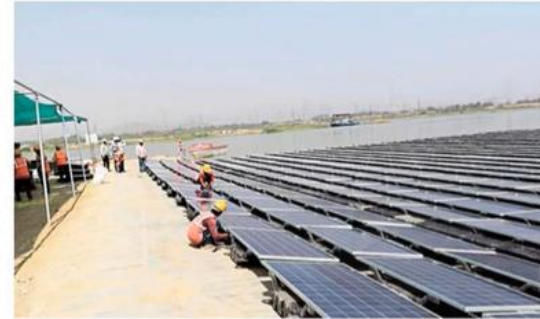
Going green: The 100 MW floating solar power plant at Ramagundam. •SPECIAL ARRANGEMENT
